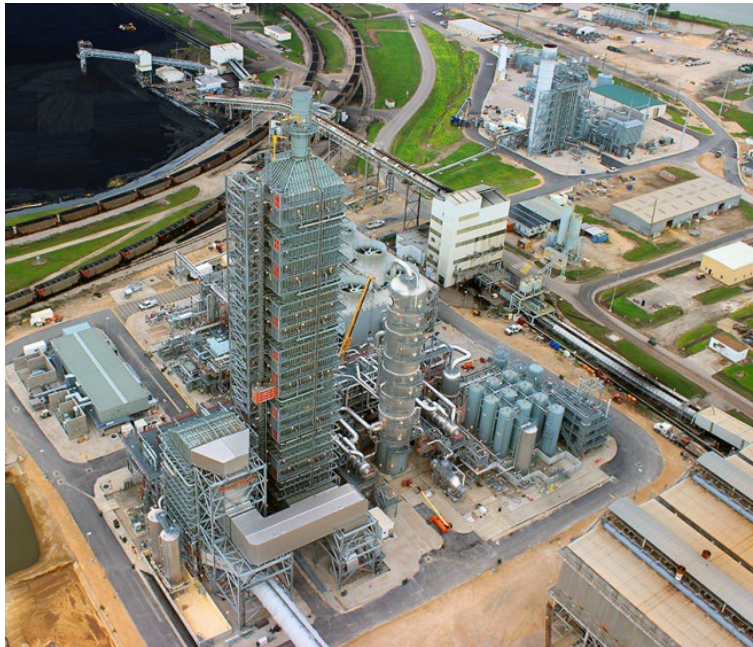
Figure 14. Petra Nova amine CC plant retrofitted to a slip stream of flue gas (equivalent to 240 MWe) from the WA Parish unit 8 coal-fired power plant. [41]
