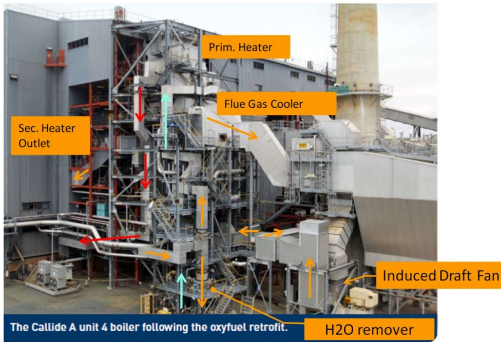
Figure 31 Photo of Callide Oxy-fuel boiler from [11] showing retrofit paths (red) and flue gas flow directions (yellow).
