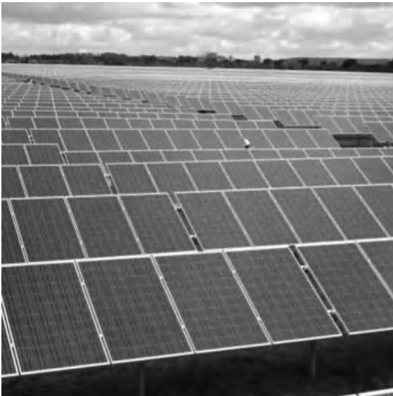
Figure 65 Conergy's 5-MW free-field system located in the parish of Hawton near Newark-on-Trent in Nottinghamshire is the largest in the UK. Photo: Lark Energy. Source: http://www.solarpowerportal.co.uk/news/conergy_completes_record-breaking_uk_solar_park/ .
