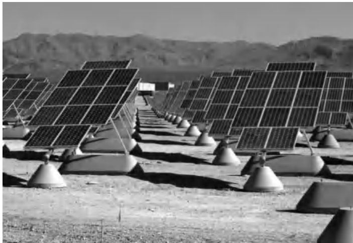
Figure 53 Photograph of the Nellis Solar Power Plant at Nellis Air Force Base; the panels track the sun in one axis. Source: http://www.nellis.af.mil/photos/media_search.asp?q=solar&btnG.x=0&btnG.y=0 .
