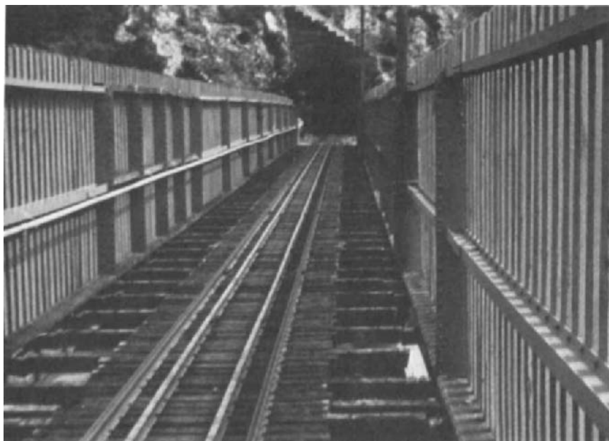
Fig. XIX.3. High bridges across valleys on the east side of the New Zealand Alps are fenced to protect trains against strong winds.
