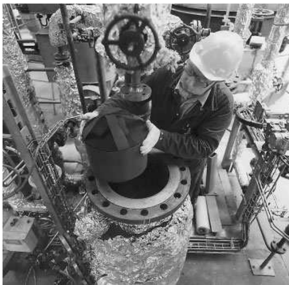
Fig. 8-7 A hydrogenation catalyst is introduced into a pilot plant in order to test it under process-relevant conditions (BASF, Ludwigshafen, Germany)
