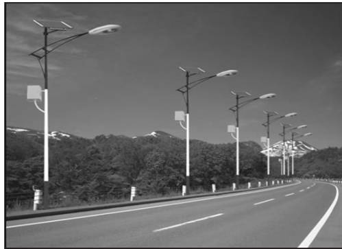
Figure 3.6 Solar street systems
