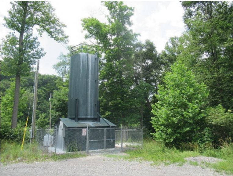
Fig. 4.2 State-owned equipment treating acid mine drainage in Birds Creek by adding powdered limestone to buffer the pH, Preston County, West Virginia, USA
