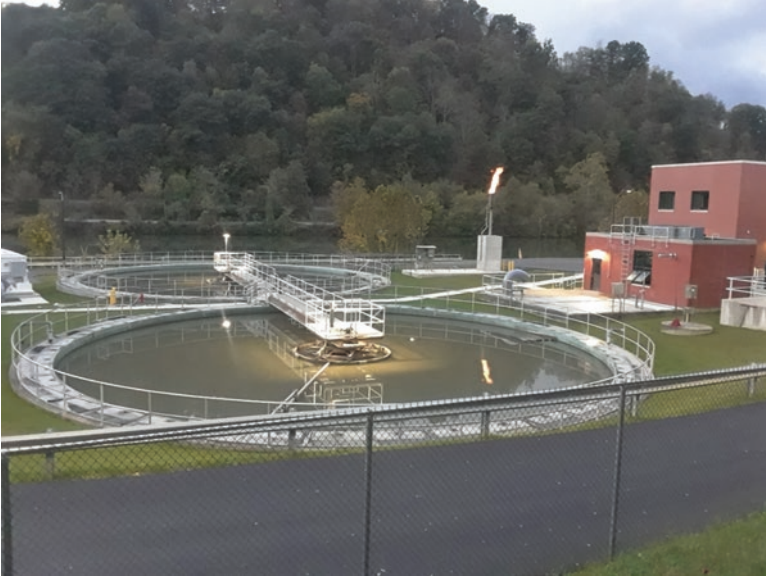
Fig. 6.3 Methane biogas being flared off (upper right) at a municipal wastewater treatment plant. (Source: Photographed in 2021 by Dan Soeder)
