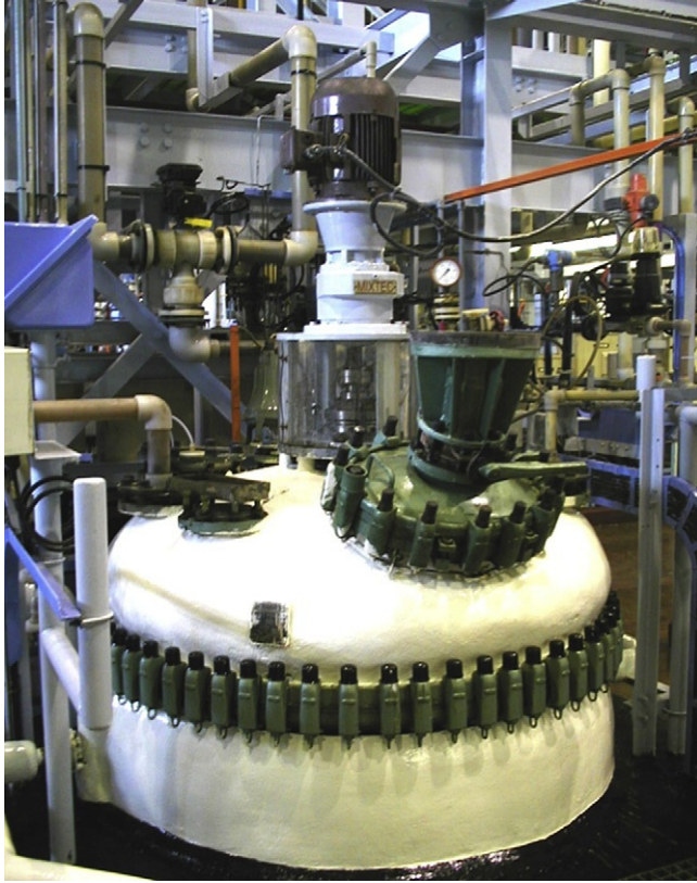
FIGURE 37.1 A Grade 2 titanium vessel used for the dissolution of a PGM concentrate. The vessel has a volume of about 2.2 m 3 . The vessel is agitated and has a heating/cooling jacket. Chlorine is intermittently passed through the contents. Photograph courtesy of Impala Platinum.
