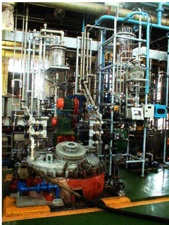
FIGURE 37.2 The ruthenium distillation section at Lonmin's Western Platinum refinery. The distillation is carried out in a glass-lined vessel. The top of this vessel is shown in the bottom center of the picture. The glass condenser can be seen in the top right. Photograph courtesy of Lonmin plc.
