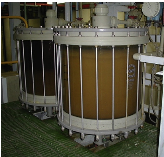
FIGURE 37.13 The ion-exchange columns used for extracting palladium from solution containing, platinum, palladium, rhodium, iridium, ruthenium, osmium and base metals, such as copper, iron and nickel. The columns are loaded with SuperLig 2, which is highly selective for palladium. The columns are small in size because the kinetics of extraction are fast. Photograph courtesy of Impala Platinum.
