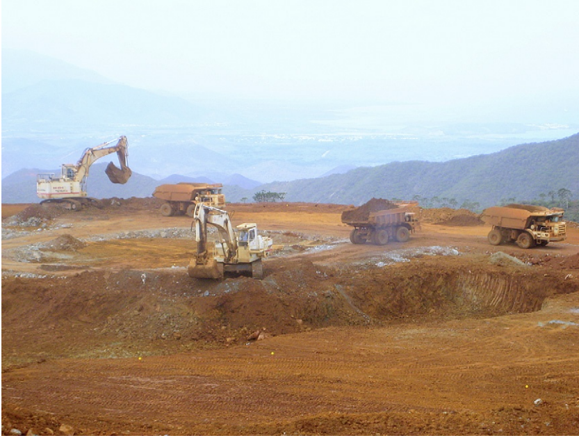
FIGURE 1.2 Hill-top laterite mine in New Caledonia. The overburden has been removed to expose the saprolite ore, which is mined as shown, upgraded and smelted to ferronickel. The ore delivered to the process plant typically contains about 2% Ni. Photograph courtesy W.G. Davenport.
