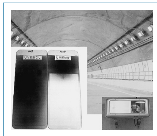
Fig.5. Glass covers on highway tunnel lighting fixtures darkened by automobile exhaust without \text{TiO}_2 and maintained clean with \text{TiO}_2 .
