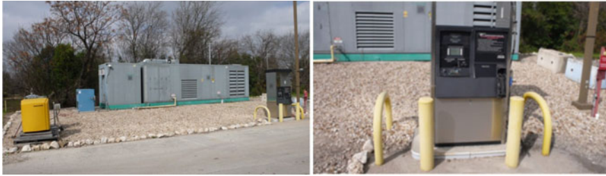
Fig. 8.1 The University of Texas at Austin SMR-based Hydrogen production, storage and Filling station. This includes many of the elements that would be expected in an example of a Small Hydrogen installation. Source Authors (WJN) with thanks to UT-Austin
