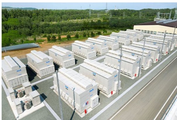
Fig. 9 High-temperature sodium–sulfur battery park for grid scale electric energy storage purpose [84] (Reprinted with permission from http://www.energy-storage.news/blogs/sponsored-ngks-nas-grid-scale-batteries-in-depth_ February 2017)
