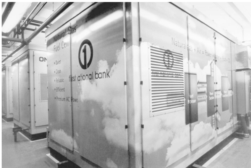
Figure 6.29: PAFC Power Plant – To the First National Bank of Omaha just a few milliseconds without electricity can mean hours of headaches and millions of dollars of lost revenues. Four UTC fuel cells 200 kW power plants now serve as the bank’s primary source of power. Heat from the fuel cell installation also provides energy for space heating, increasing the overall efficiency of the fuel cell system to more than 80%.
