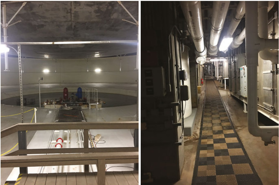
Figure 11.19: Environment and climate management infrastructure in the basement of Biosphere 2. (Left) The mechanical “lung” and (right) one of the basement hallways with tubing and piping infrastructure for climate management in Biosphere 2.
