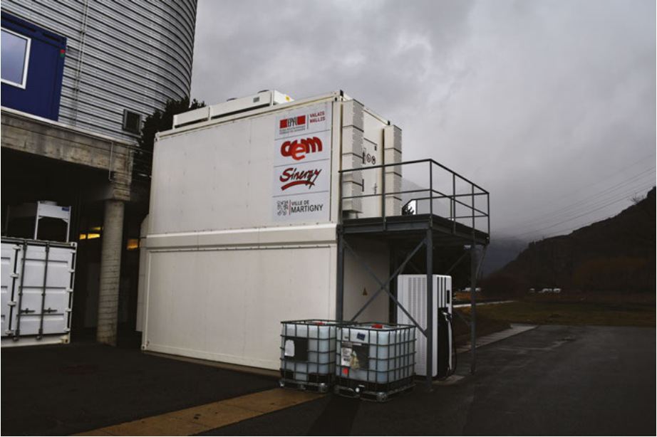
Figure 4.32: Vanadium-based redox flow battery plant at the EPFL research lab in Martigny, Switzerland. The two large white containers feed that fast electric charging terminal for electric vehicles. 200 kW/400 kWh Vanadium Redox Flow Battery connected to a 80 kW charger in Martigny. Photo by Artur Braun, 7 March 2018.
