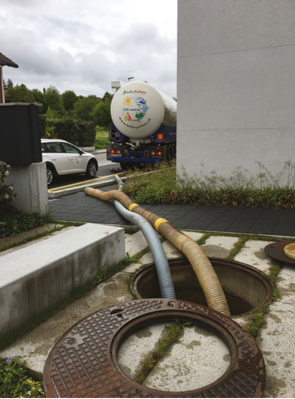
Figure 9.12: Two hoses right before connection to the pellet delivery truck, one of which blows the pellets into the pellet storage container in the basement of the residential home. The second hose sucks air from this storage container in the basement so as to remove wood dust.
