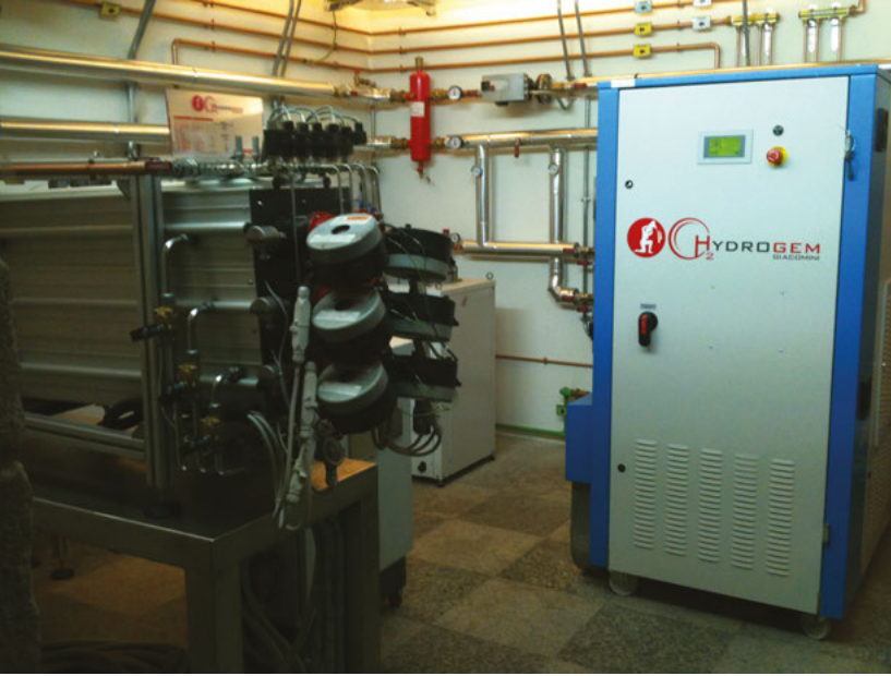
Figure 1.15: The Giacomini H 2 YDROGEM system installed in the ground floor of a residential home in Orta San Giulia, Novarra, Italy.
