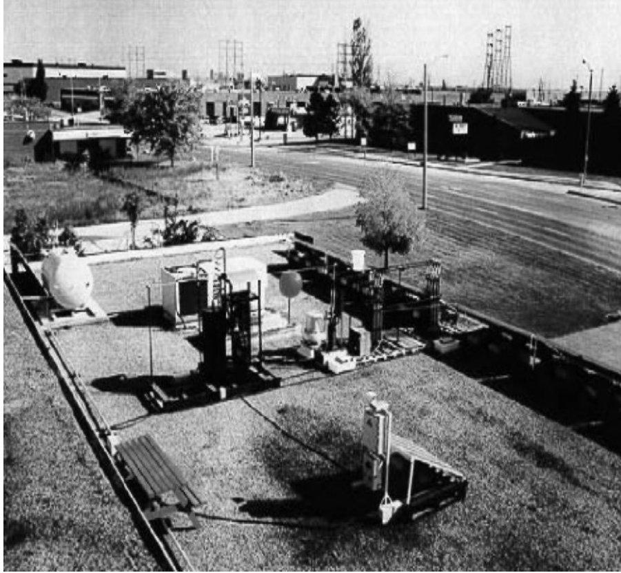
Fig. 49: The Alexander T. Stuart renewable energy test site
